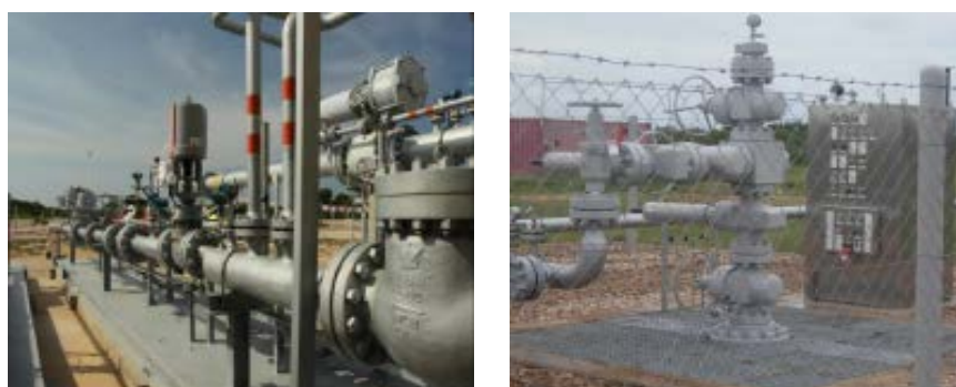
Kiliwani North facilities and wellhead, Tanzania
